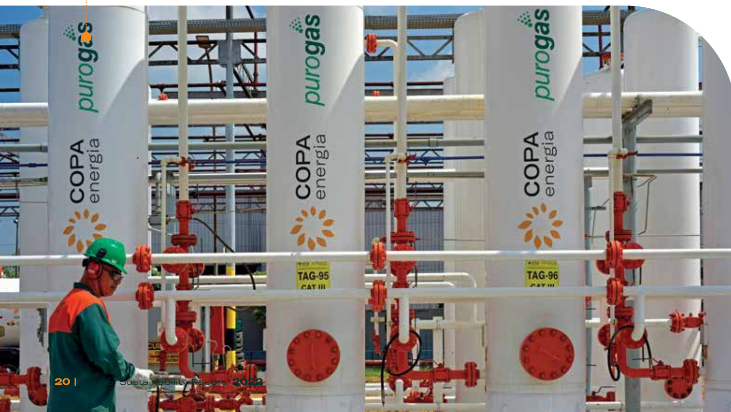
Jeferson Damaceno Garcia checking the tanks of Purogas in the CO of Capuava.
